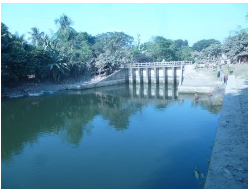
Photograph 3.3: The newly constructed regulator (BWDB design) close to water structure (British design) at the mouth of Kata Khal joining the Kobadak River at Jhikargacha.
